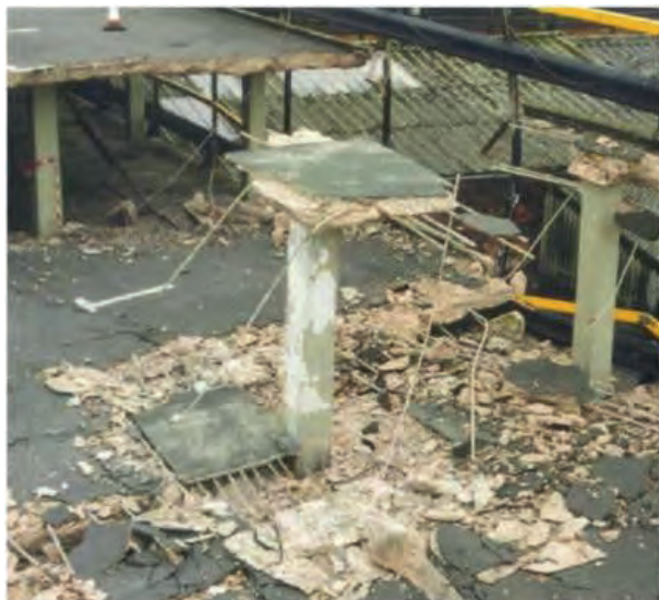
Figure 1. Punching failure of a flat slab from [ http://civildigital.com/punching-shear-punching-shear-flat-slabs/ ]
