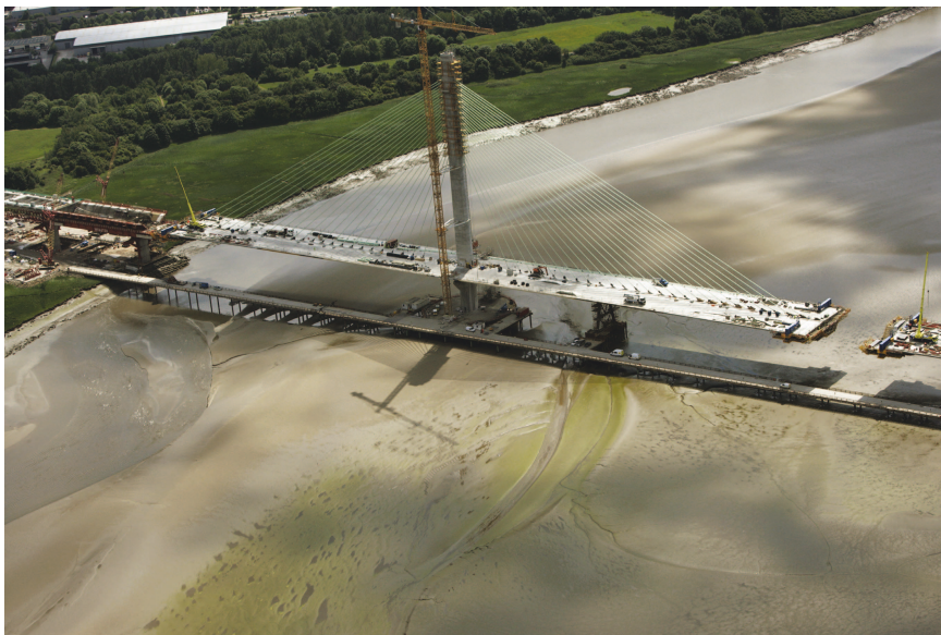
Figure 6.2: Mersey Gateway Bridge: south tower in the erection stage, including the temporary pier that was not considered in this study (picture courtesy Halton Borough Council, from www.merseygateway.co.uk ).
